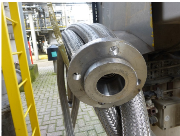
Figure 6: Flexible steel hose for connecting the cooling circuit with interim storage tank during maintenance
