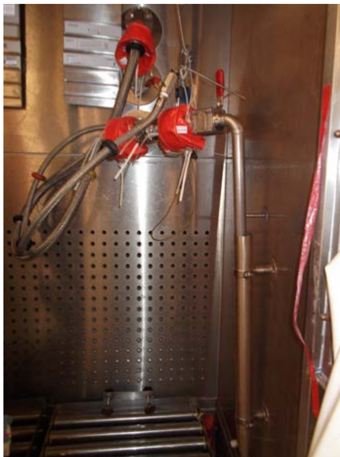
Figure 2: Suction lance inside the containment booth, with connected piping and storage drum
